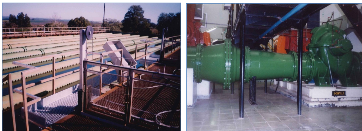
Figure 5: The CCT's Water Treatment Works and Low Lift Pumps at Voëlvlei Dam
