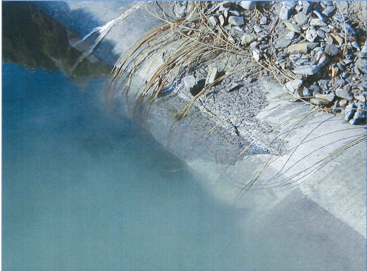
Figure 30 Typical Pipe Burst on the CCT's Potable Water Pipeline from the Voëlvlei Dam
